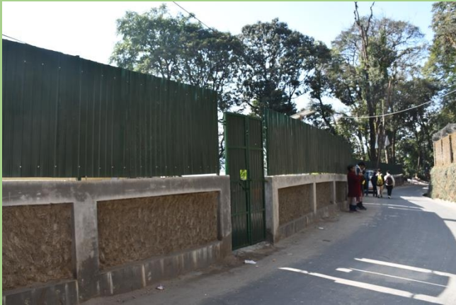
Fig: Extension of boundary wall around the staff quarter compound at PNHZ Park
